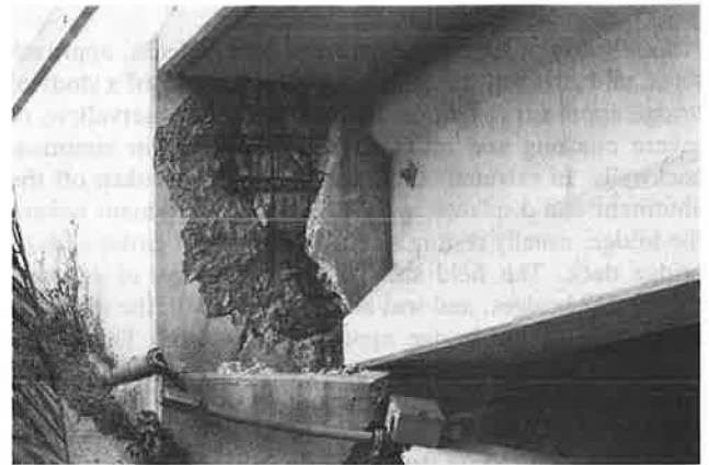
FIGURE 5 Observed abutment backwall damage, advanced stage.
