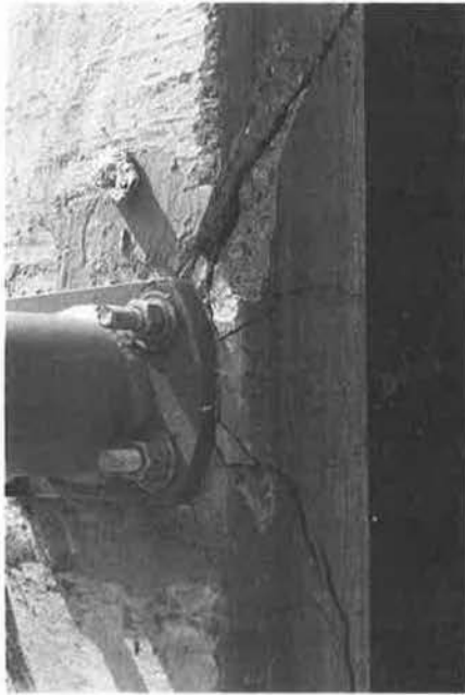
FIGURE 12 Damage at Post 5.
