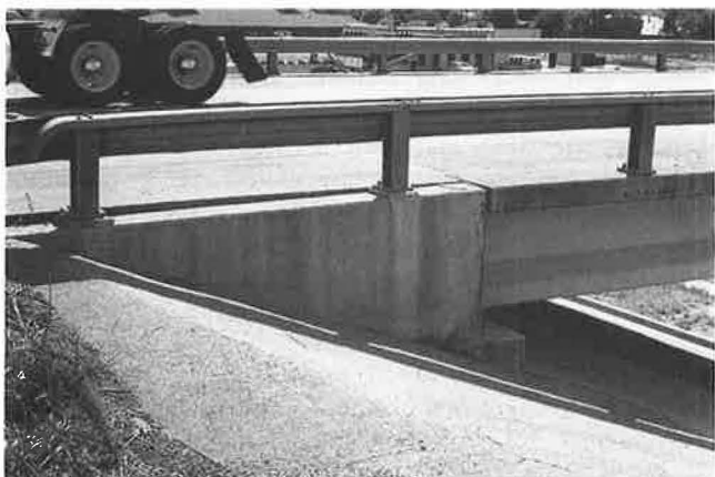
FIGURE 7 Observed damage to abutment wingwall at structure adjacent to ACP: Case 2.
