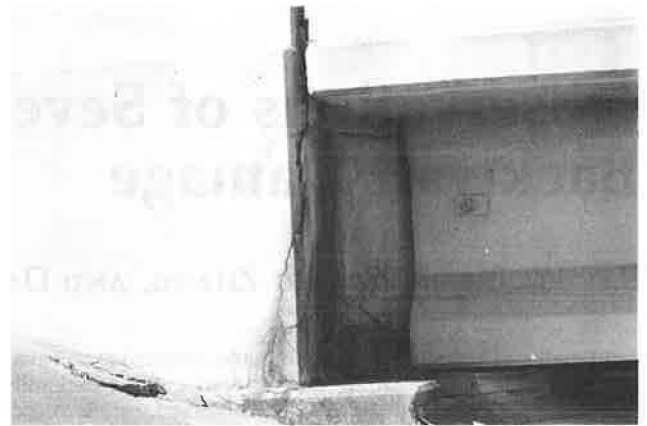
FIGURE 4 Observed abutment backwall damage, intermediate stage.
