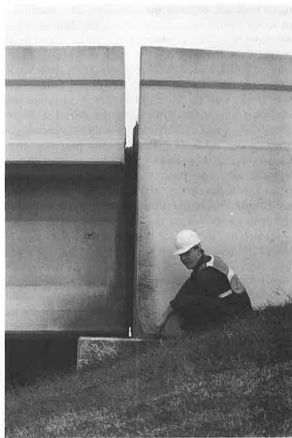
FIGURE 9 Rotated abutment and wingwall.
