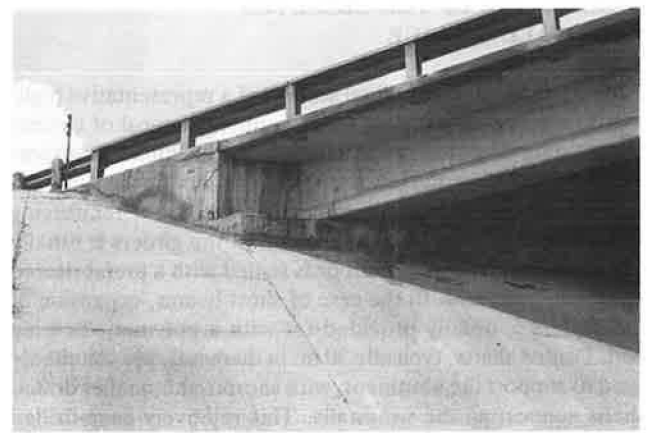
FIGURE 6 Isolated instance of observed damage to abutment backwall adjacent to ACP.
