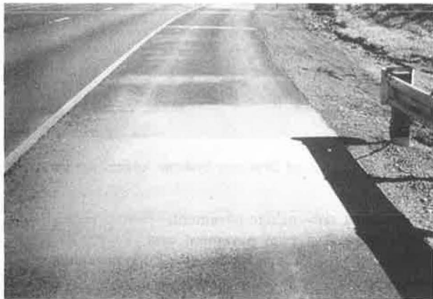
FIGURE 6 Site of Test Pit 1: severe staining of shoulder.
