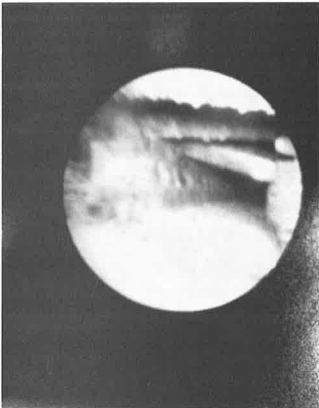
FIGURE 8 Partially misshapen inner core of Type-A edge drain.
