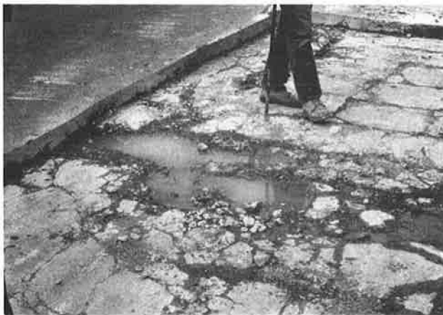
FIGURE 11 Water ponding in old broken slab.
