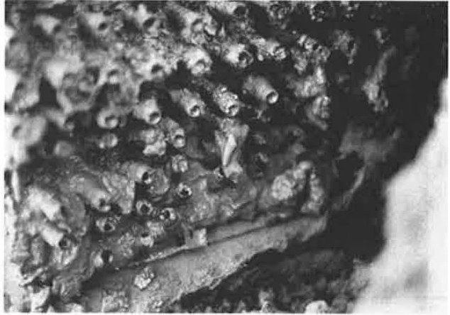
FIGURE 16 Exposed inner core showing siltation.
