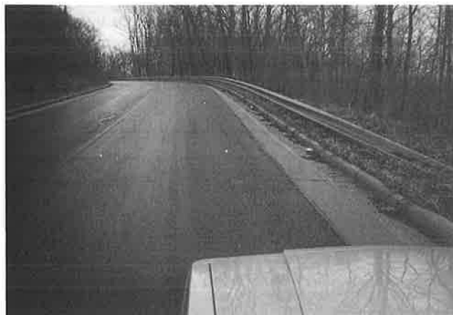
FIGURE 13 Condition of pavement on typical curbed section.
