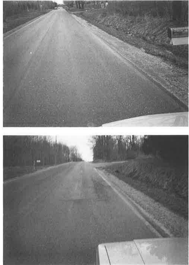
FIGURE 17 Condition of pavement on typical uncurbed section east of spring area, two views.
