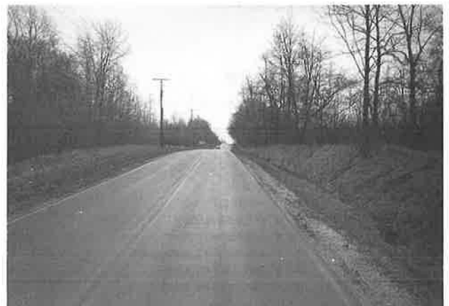
FIGURE 15 Condition of pavement in spring area.
