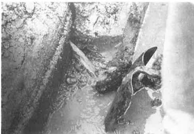
FIGURE 10 Water flow from hydraway, Test Pit 2.
