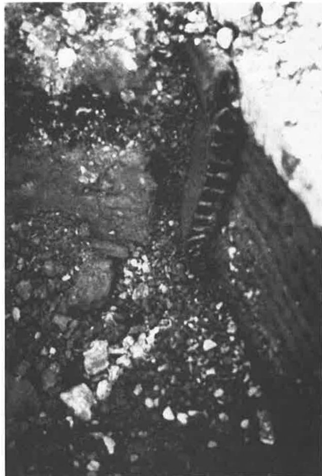
FIGURE 3 Excavated geocomposite showing similar fabric intrusion to that in Figure 2.
