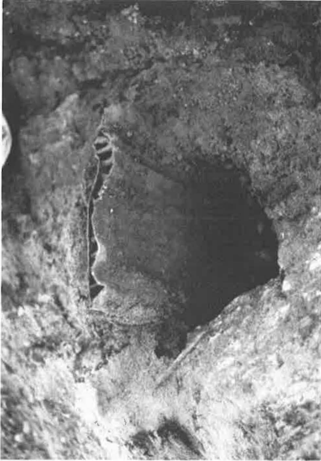
FIGURE 14 Severely compressed Type-A drain.
