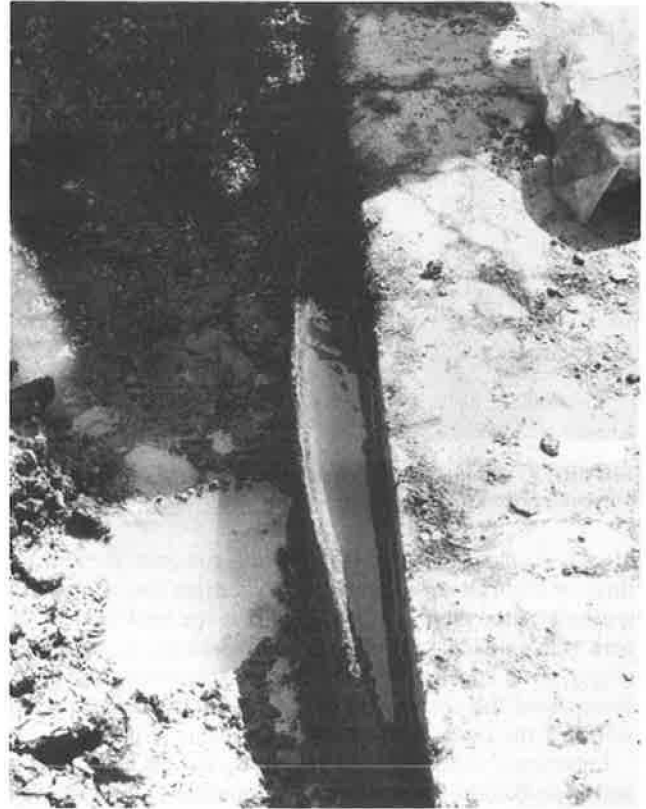
FIGURE 12 Water ponding behind Type-A edge drain.
