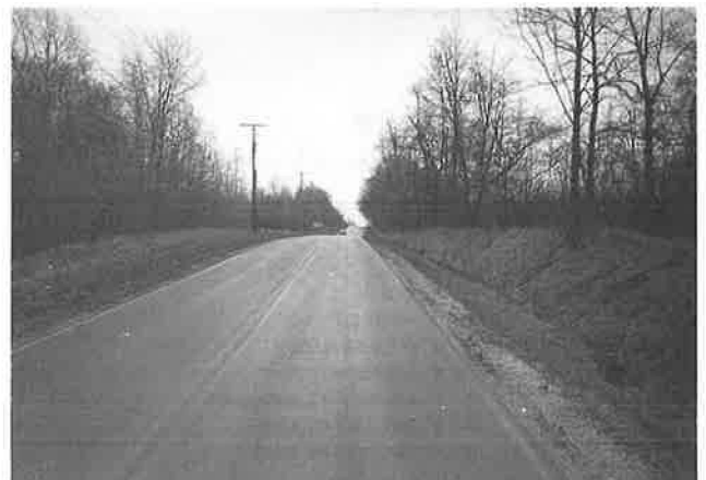
FIGURE 15 Condition of pavement in spring area.
