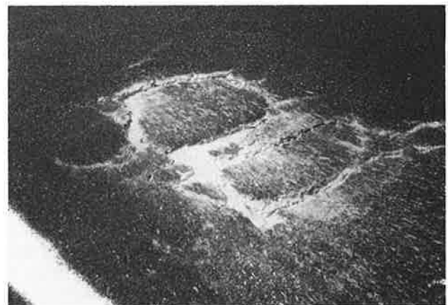
FIGURE 9 Water and silty fines pumping up through pavement on Pennyrile Parkway.
