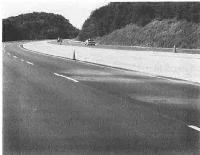
FIGURE 21 Silt being pumped up at centerline of Mountain Parkway.
