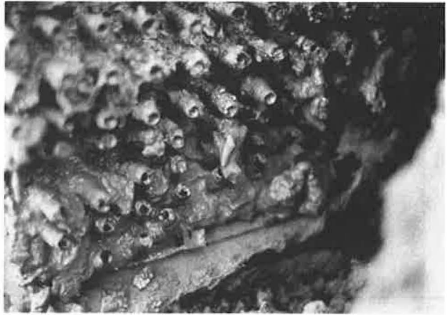
FIGURE 16 Exposed inner core showing siltation.
