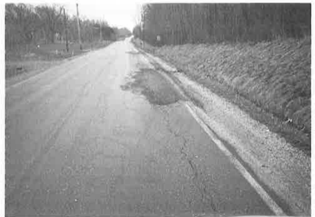
FIGURE 14 Condition of pavement on typical uncurbed section west of spring area.
