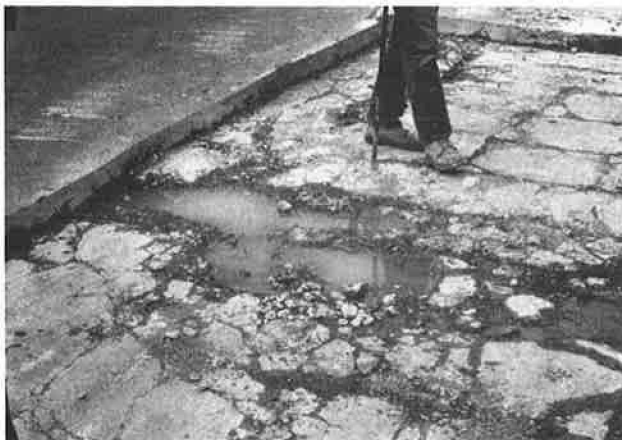
FIGURE 11 Water ponding in old broken slab.
