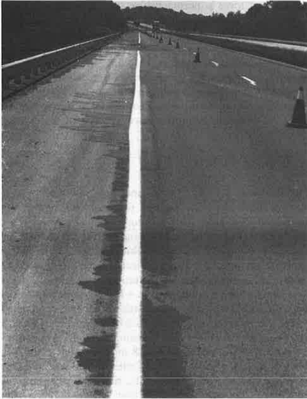
FIGURE 10 Water pumping up through asphalt overlay directly above edge drain.
