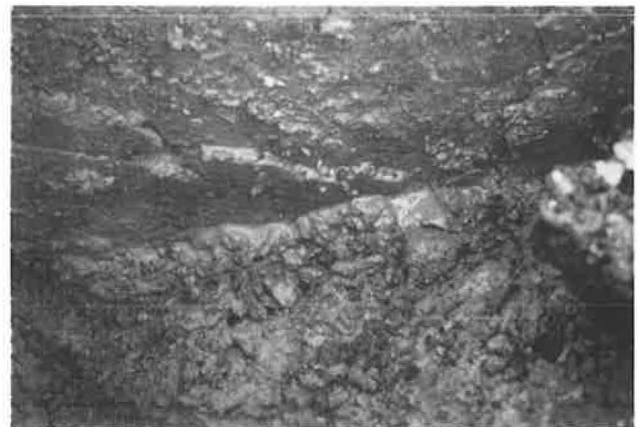
FIGURE 8 Free water from cracked pavement slab, Test Pit 1.
