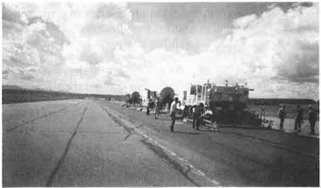
FIGURE 5 Heat reforming process (HRP-6) on Runway 15-33 at Prince George Airport (50 mm with rejuvenation, remix option) (9,10).
