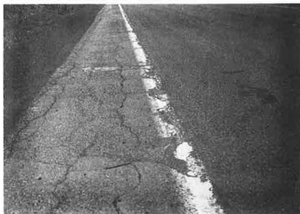
FIGURE 3 Lava Springs–Sand Shed, May 1990. Nonrecycled shoulder on left and recycled travel lane on right.
