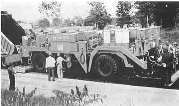
FIGURE 2 Heat reforming process (HRP-5) on Ontario Highway 5/24, showing reformer (40 mm with rejuvenation, remix option) (7).
