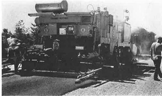
FIGURE 4 Heat reforming process (HRP-6) on British Columbia Highway 1 near Langley (40 mm without rejuvenation, reform option) (8).
