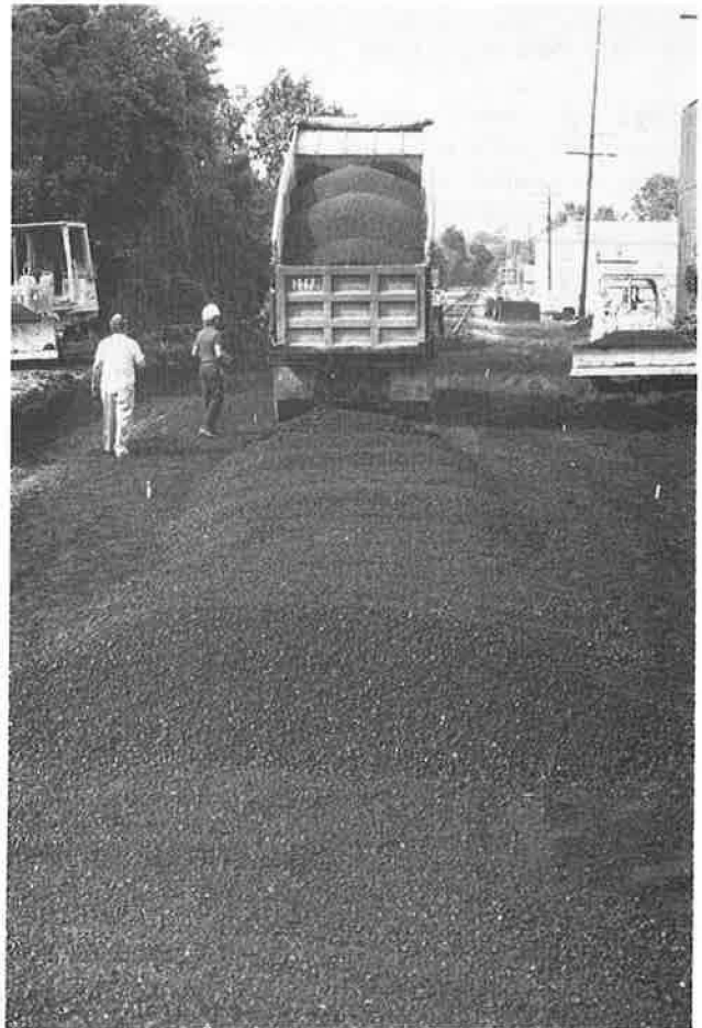
FIGURE 3 Placement of HMA with paver ( top ) and backdumping and spreading with dozer ( bottom ).
