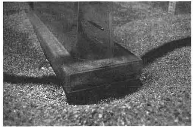
FIGURE 3 Scour hole observed without monitoring device.
