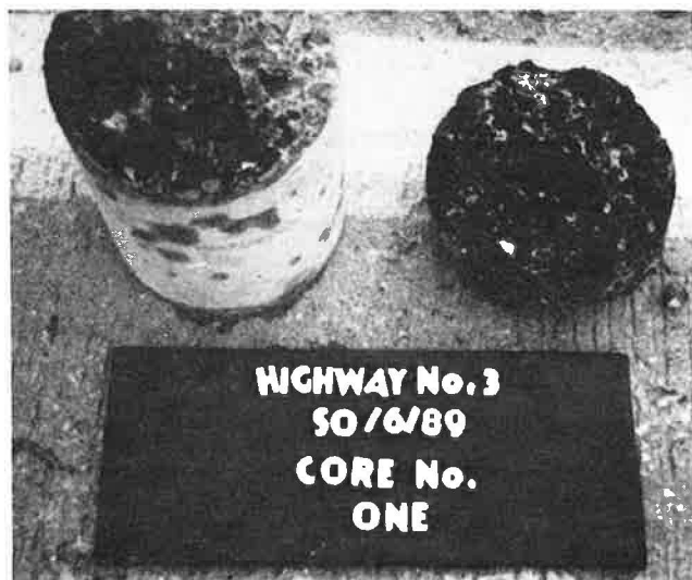
FIGURE 4 150-mm core obtained from cracks or joints, Highway 3N. OGDL material basically in one place and partially bonded to surface layer.
