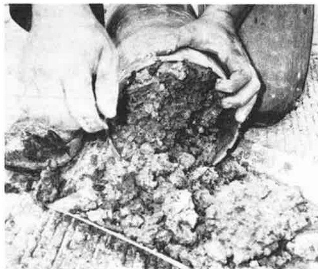
FIGURE 5 150-mm core obtained at transverse joint, Highway 3N. OGDL material loose mixture of stripped OGDL aggregate particles and subgrade soil.
