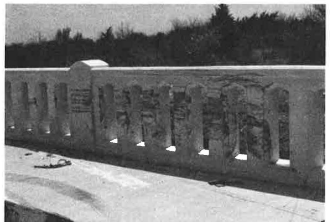
FIGURE 15 Bridge rail after Test 1185-6.
