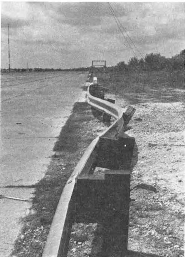
FIGURE 8 Photographs of damage to test installation after Test 7147-5.
