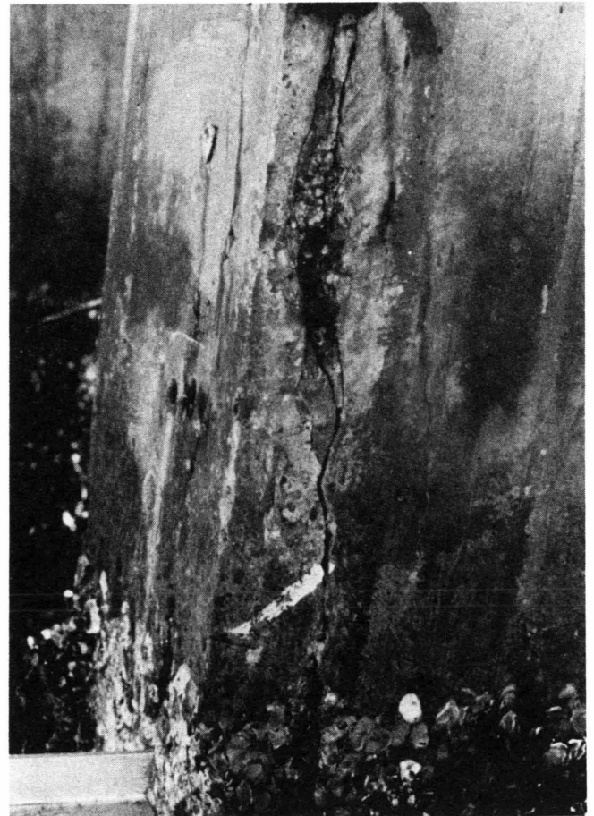
FIGURE 1 Excessive vertical cracking and spalling of concrete in a pile (B. B. McCormick Bridge, Jacksonville).
