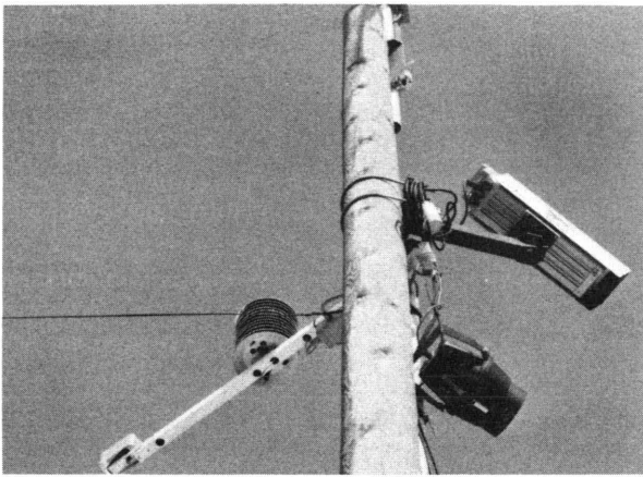
FIGURE 22 Camera control post in connection of a road weather station. The camera has infrared light for night use.
