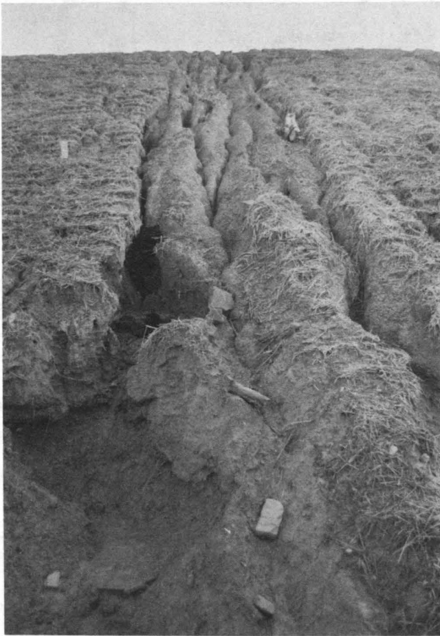
FIGURE 3 Gullies, rills, and tunnels on 2:1 slope.
