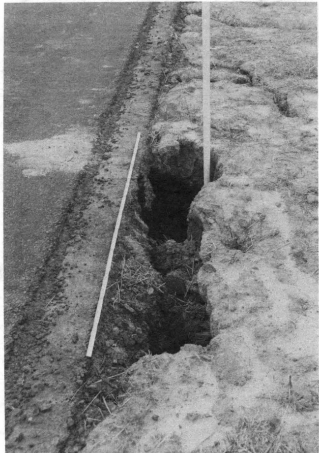
FIGURE 2 Formation of jugs near pavement edge.
