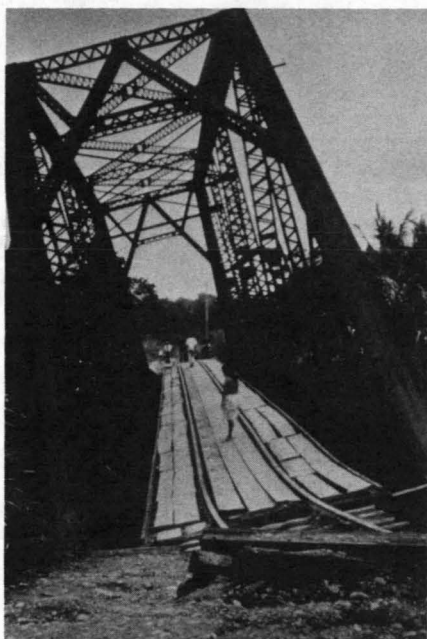
FIGURE 10 Railway bridge over the Rio Bananito that tipped during the 1991 Costa Rican earthquake; lateral ground displacement pushed the supporting caissons from the bridge seatings leaving the truss unsupported (photograph courtesy of Laboratorio de Ingenieria Seismica de la Universidad de Costa Rica).
