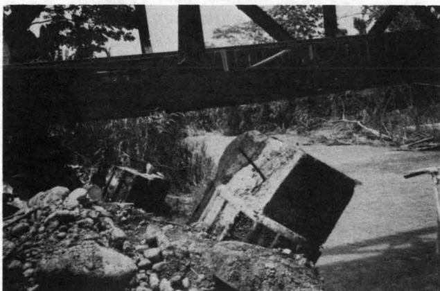
FIGURE 11 Caissons beneath the Rio Bananito railway bridge that were pushed riverward by lateral ground displacement during the 1991 Costa Rica earthquake (photograph by T. L. Youd).
