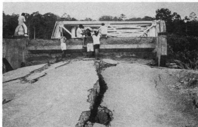
FIGURE 13 Liquefaction-induced settlement and deformation of approach fill adjacent to southern abutment of Rio Estrella highway bridge (photograph courtesy of Laboratorio de Ingenieria Seismica de la Universidad de Costa Rica).
