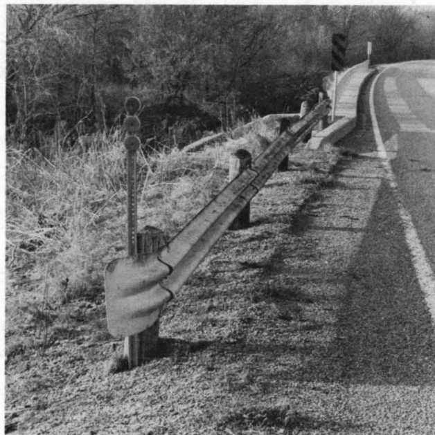
FIGURE 1 Example of typical exposed guardrail end.
