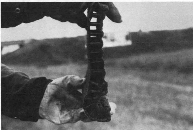
FIGURE 13 View of J-buckling in exposed fin drain.
