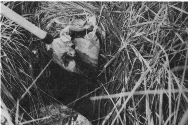
FIGURE 7 View of crushed outlet pipe.
