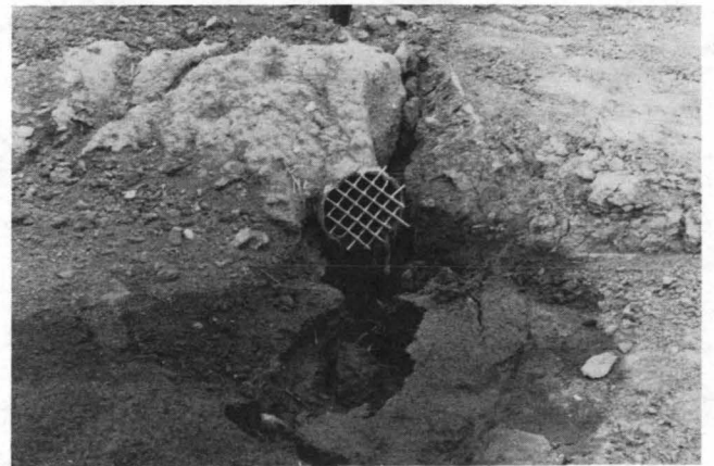
FIGURE 9 Erosion around newly constructed outlet pipe.
