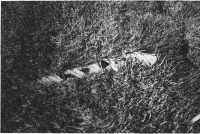
FIGURE 6 View of exposed and damaged outlet pipe.
