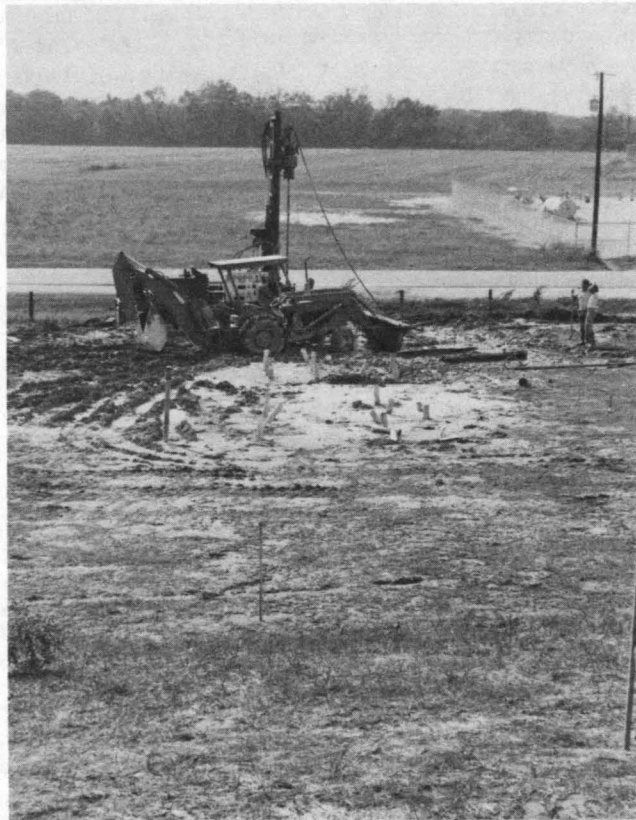
FIGURE 5 Westward-looking views of the HDD drill rig setup site after carrier pipe pull-in. Top , drilling mud seeps mixed with grout returns from the directional borehole immediately after completion of the crossing. Bottom (foreground), jet grouting through the levee's seepage retardation berm. The purpose of the grouting, completed almost 1 year after line pull-in, was to help ensure viability of the soil-pipe annulus plug. Note effectiveness of site surface cleanup efforts ( bottom , background).
