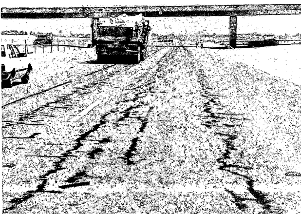
FIGURE 5 Typical alligator cracking in SEA Section B of Test Road 2 (Abu Hadriyah Expressway).
