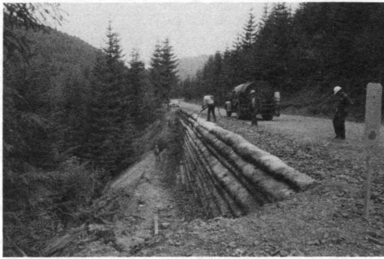
FIGURE 1 Geotextile wall, with exposed material being sprayed with emulsified asphalt after construction.
