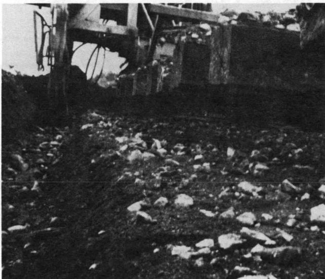
FIGURE 3 Condition of undercut ballast surface showing protruding particles.
