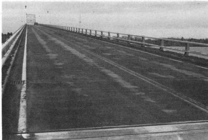
FIGURE 4 "Washboard" deterioration on Crown Point Bridge.
