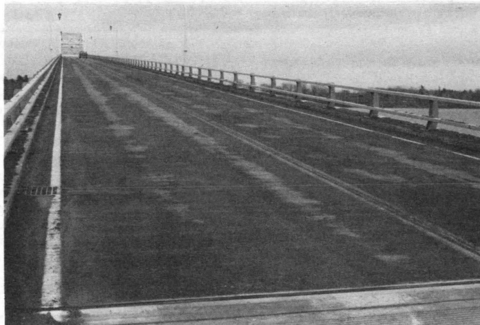
FIGURE 4 "Washboard" deterioration on Crown Point Bridge.
