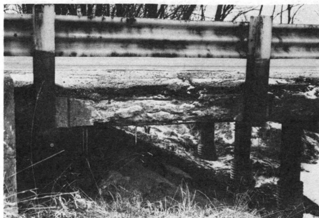
FIGURE 2 Damage in shoulder of Bridge 2.
