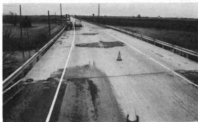
FIGURE 3 Patched regions over pier lines in deck of Bridge 3.
