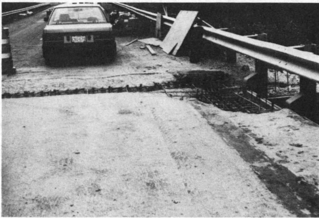
FIGURE 4 Cuts through deck of bridge 1 at abutments.
