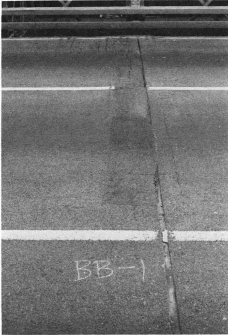
FIGURE 3 Cracking at relief joint has been patched.
