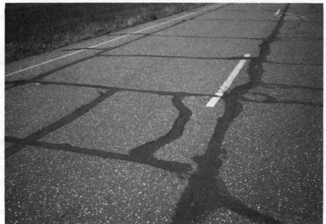
FIGURE 1 Reflective cracking typical of test site location.
