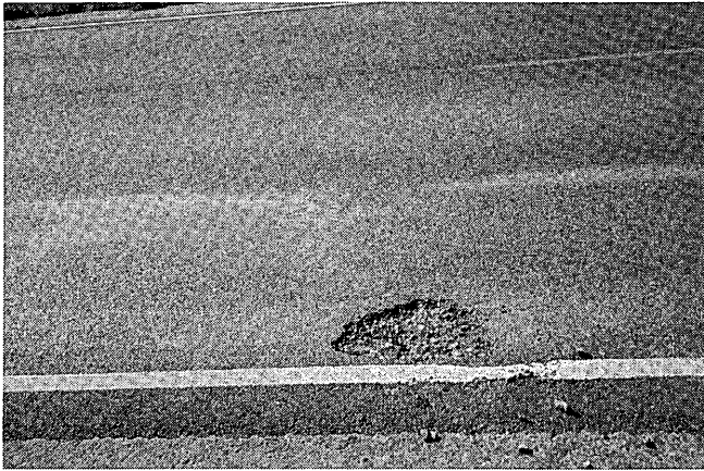
FIGURE 2 Three stages of stripping: white spots, fatty area, and pothole (close up).
