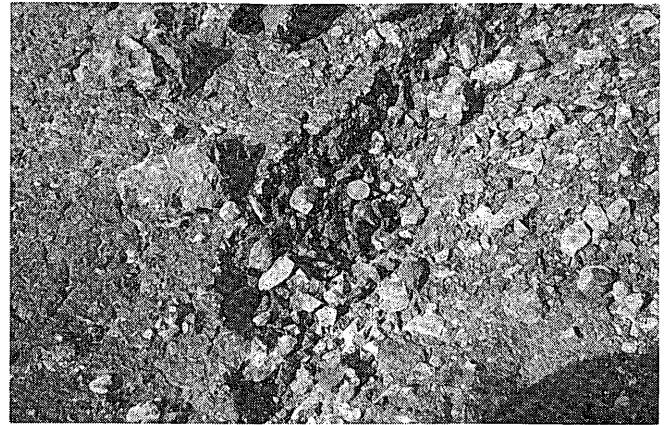
FIGURE 4 Close up of pothole showing severely stripped aggregate.
