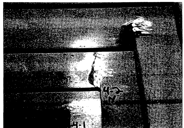
FIGURE 3 Crack in centerbeam at toe of stirrup weld.
