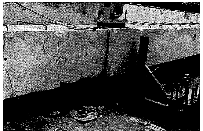
FIGURE 10 Crack pattern for deteriorated beam just before failure.
