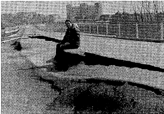
FIGURE 7 Drops of 2 to 3 ft on one side of UWLS ramp, February 1983.
