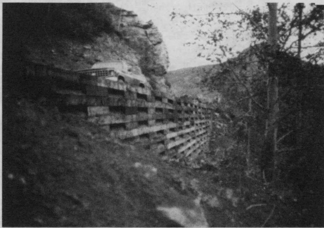
FIGURE 2 Timber-faced geogrid-reinforced wall in forest setting constructed with native soil backfill (San Juan National Forest, Colorado).
