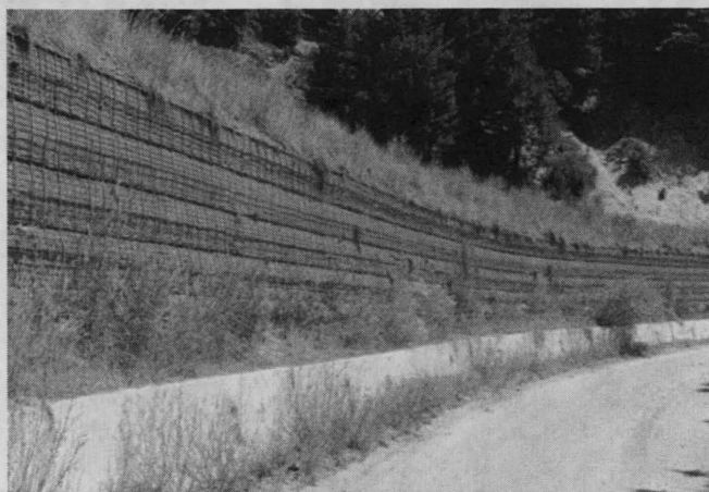
FIGURE 1 Seven-year-old welded wire wall with some face settlement due to use of native soil backfill (Plumas National Forest, California).
