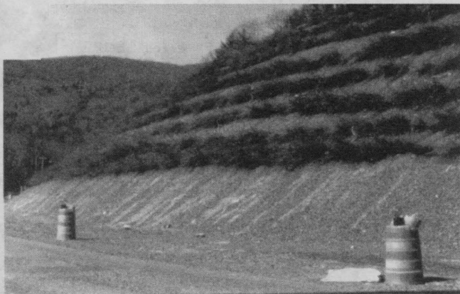
FIGURE 4 Brush-layer buttress fill immediately after construction (winter 1990, Greenfield Road, near Route 112, Colrain, Mass.).
