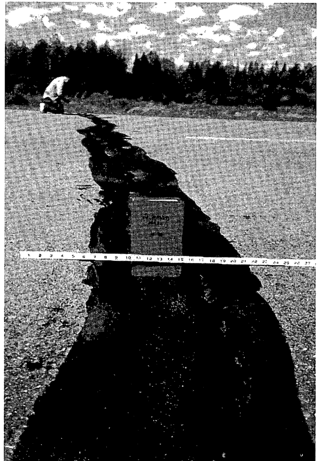
FIGURE 9 Transverse runway crack.
