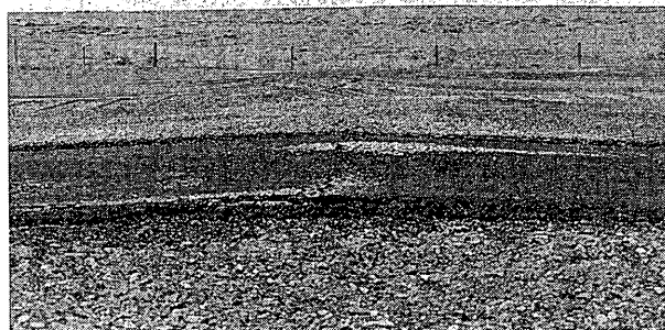
FIGURE 1 Damaged pavement sections after milling.
