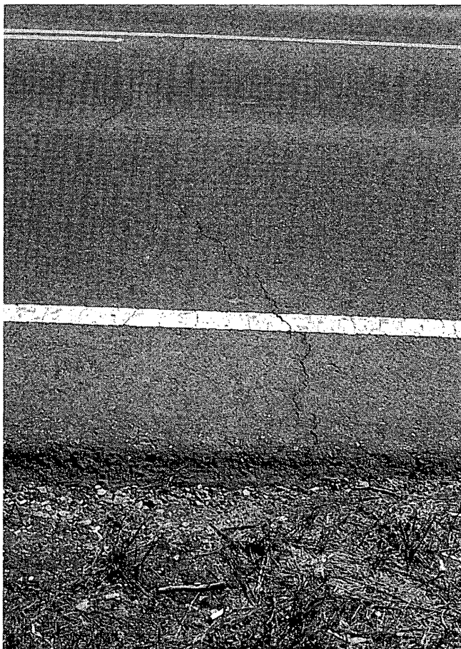
FIGURE 5 Typical transverse crack.
