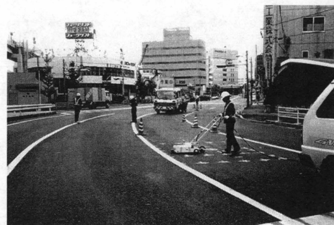
FIGURE 8 Void area on a city street isolated by portable GPR units and marked with spray paint.
