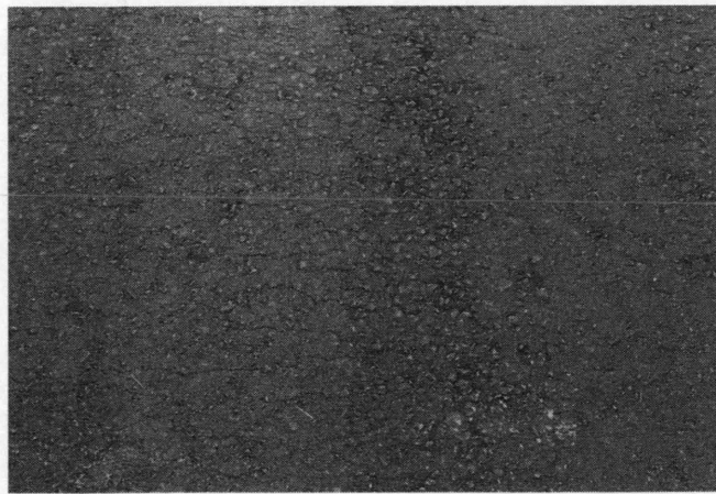
FIGURE 2 Segregation streak on surface.
