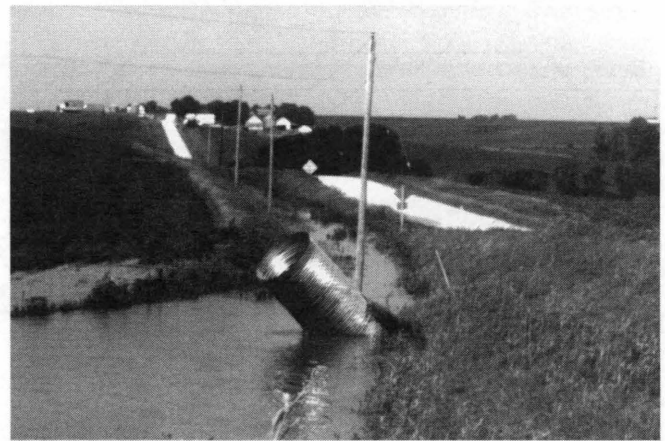
a. FAILED CMP WITHOUT TIE-DOWN SYSTEM.
