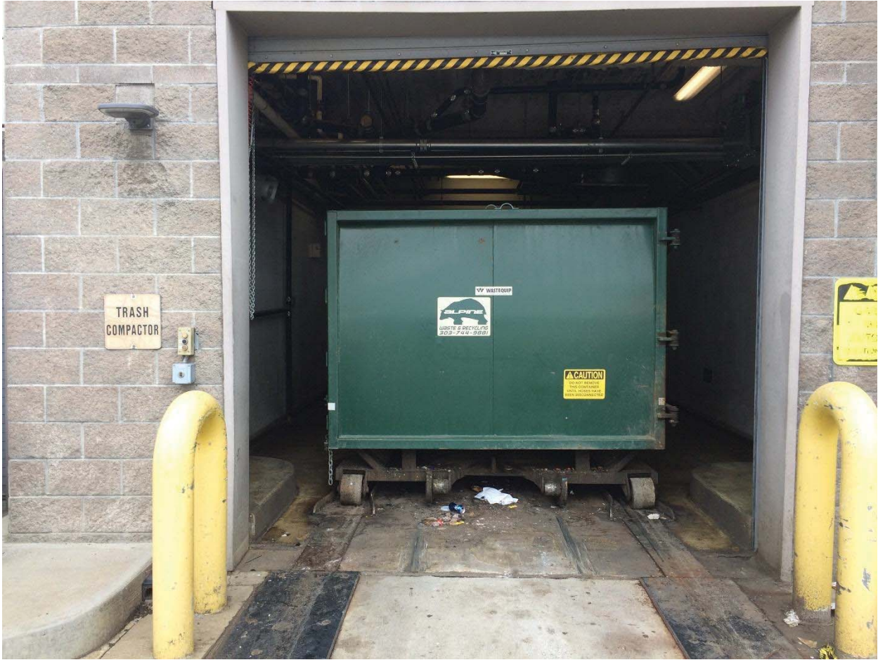
Figure 3: Terminal concourse trash compactor, courtesy of Denver International Airport
