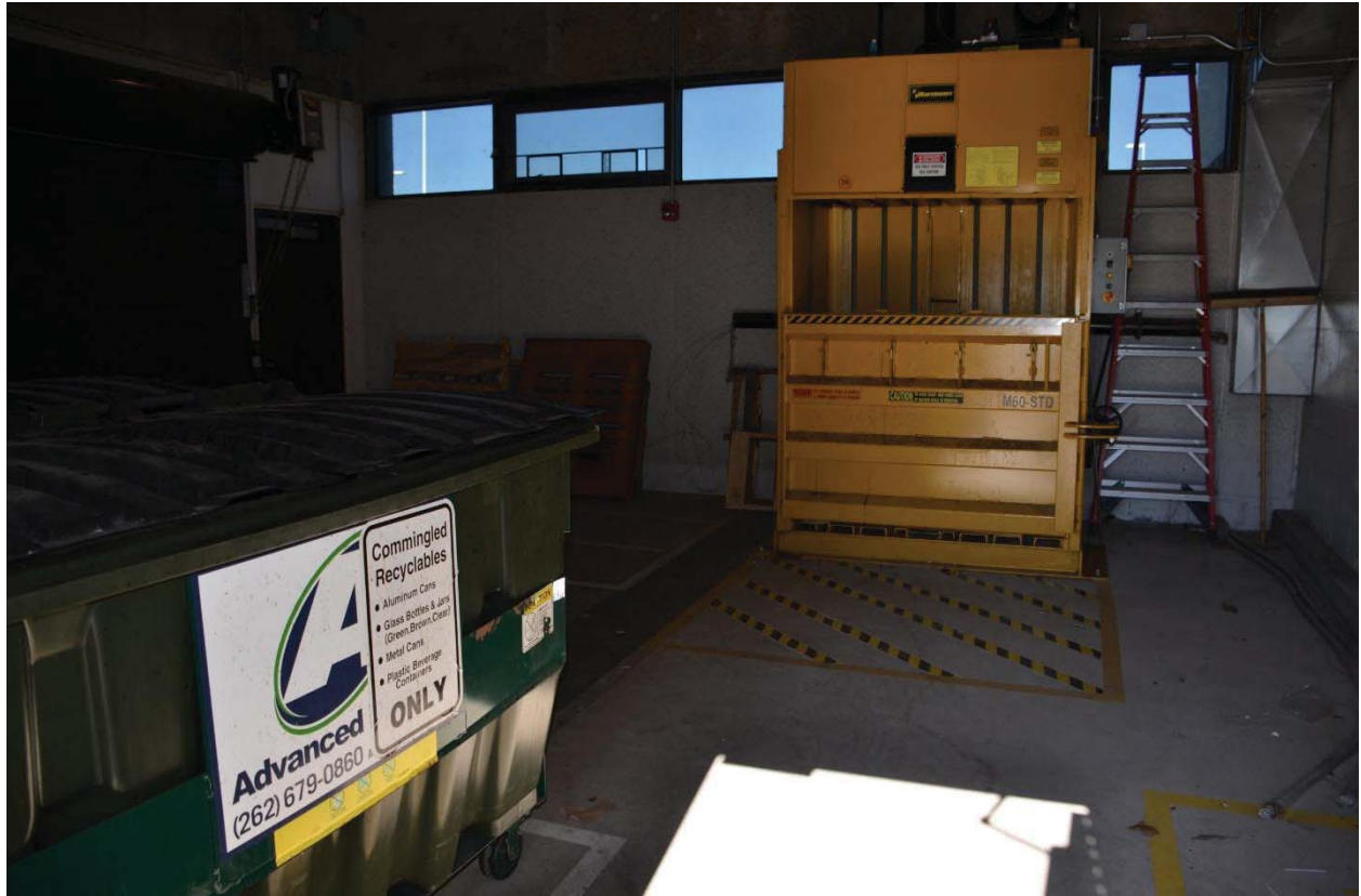
Figure 7: Commingled recycling dumpsters and cardboard baler in airside recycling area; courtesy of County of Milwaukee Airport Division
