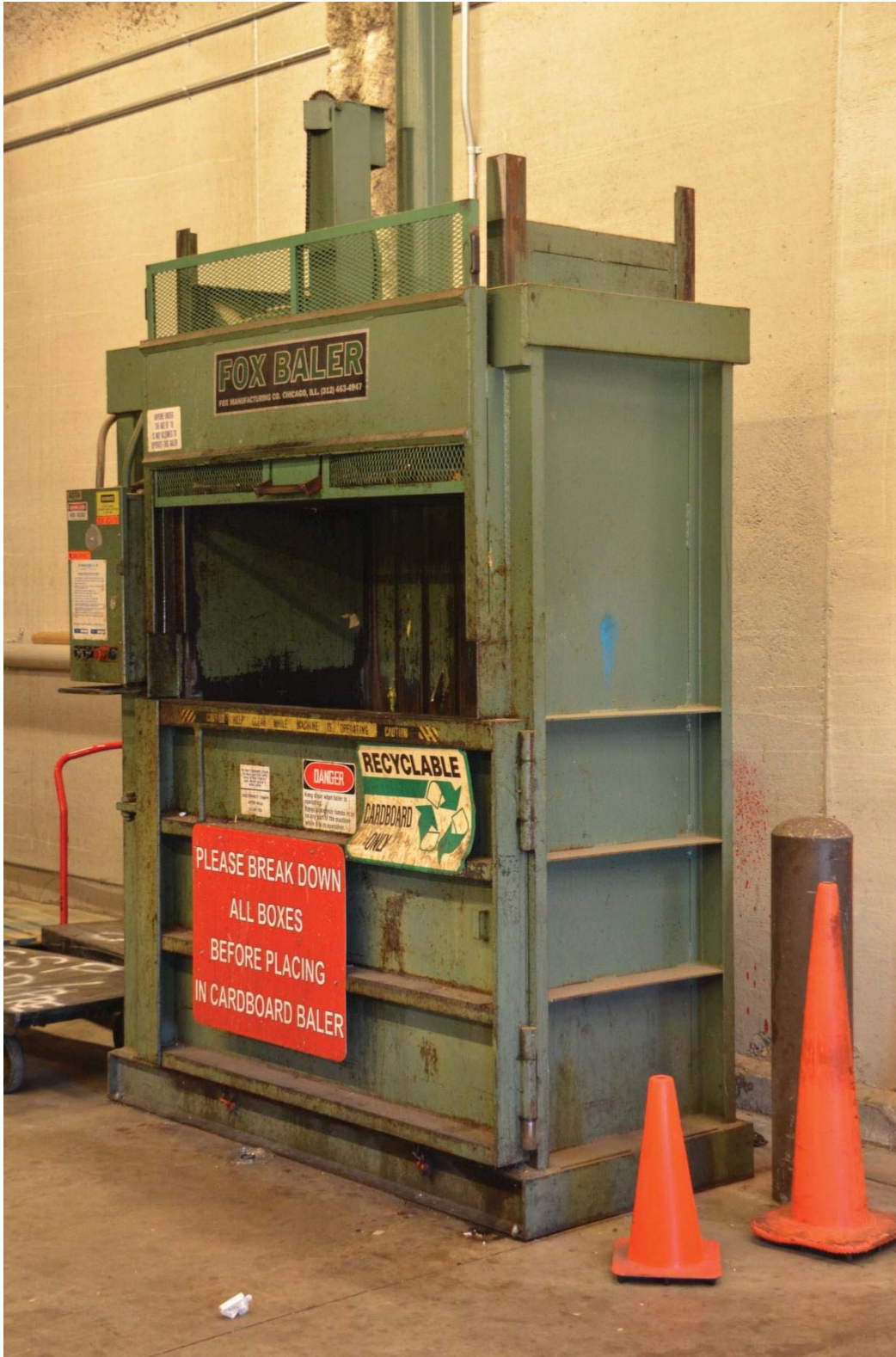
Figure 4: Cardboard baler; courtesy of County of Milwaukee Airport Division
