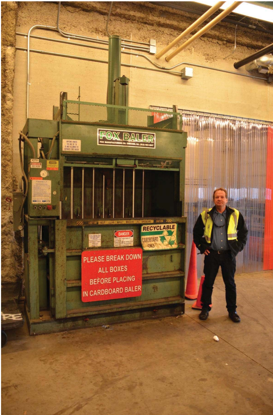
Figure 3: Cardboard baler; courtesy of County of Milwaukee Airport Division
