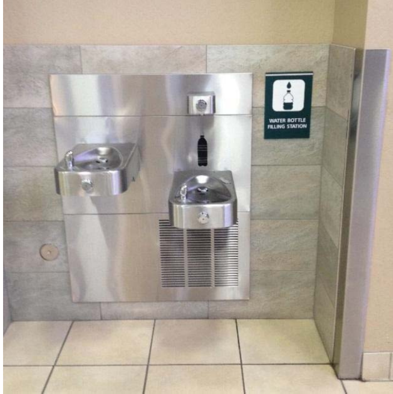
Figure 2: Terminal Drinking Fountain and Water Bottle Filling Station, courtesy of Reno-Tahoe International Airport
