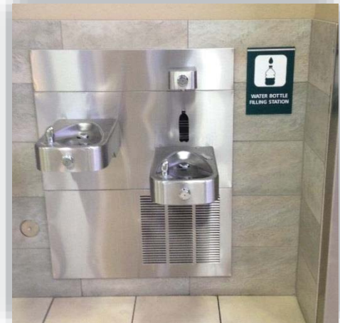
Figure G-6: Drinking Fountain/ Water Bottle Filling Station in Passenger Terminal
