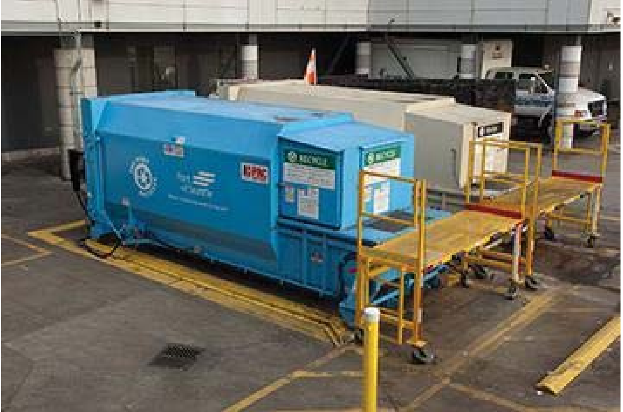
Figure 4: Side by side waste and recycling compactors; courtesy of Port of Seattle
