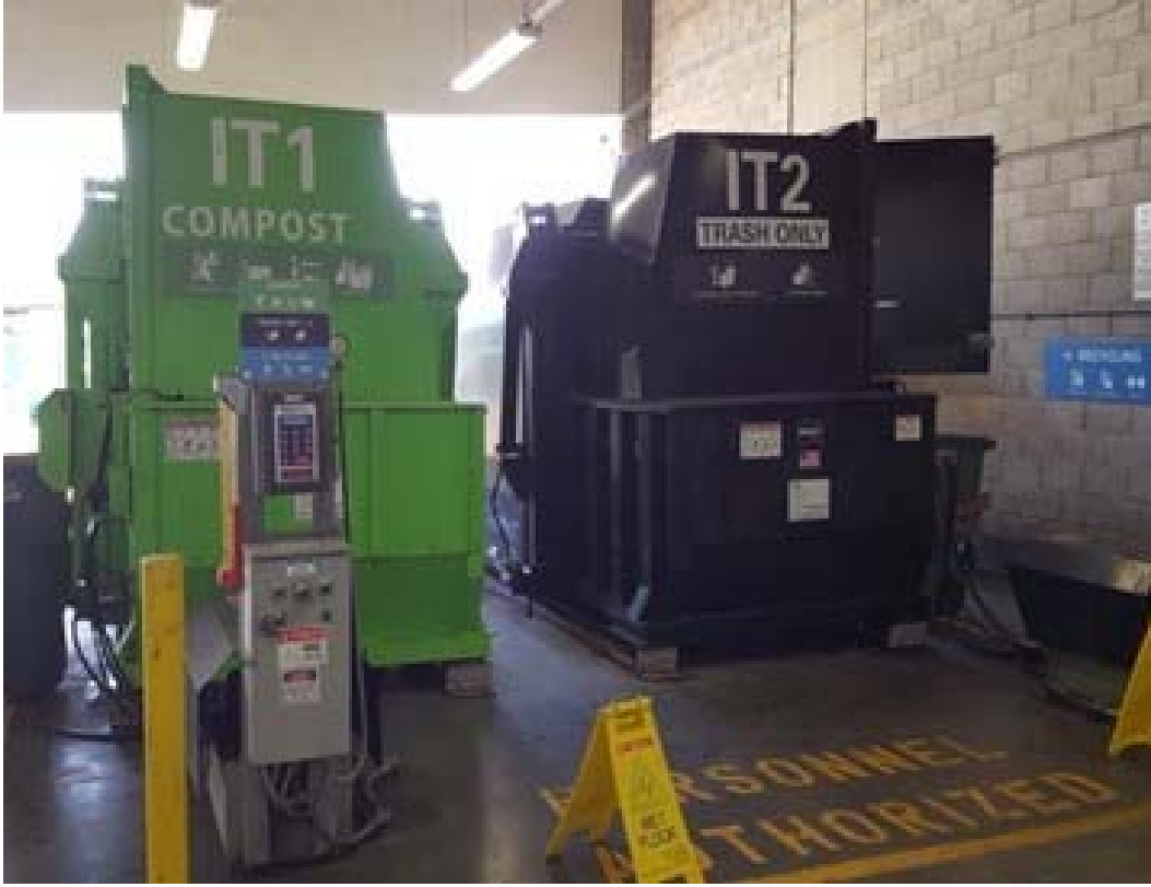
Figure 8: Standard signage on Materials Recovery Area compactors; courtesy of San Francisco International Airport
