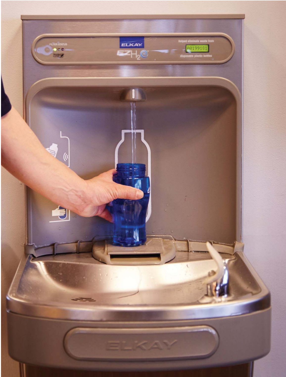
Figure 11: Terminal bottle filling station; courtesy of Salt Lake City Department of Airports
