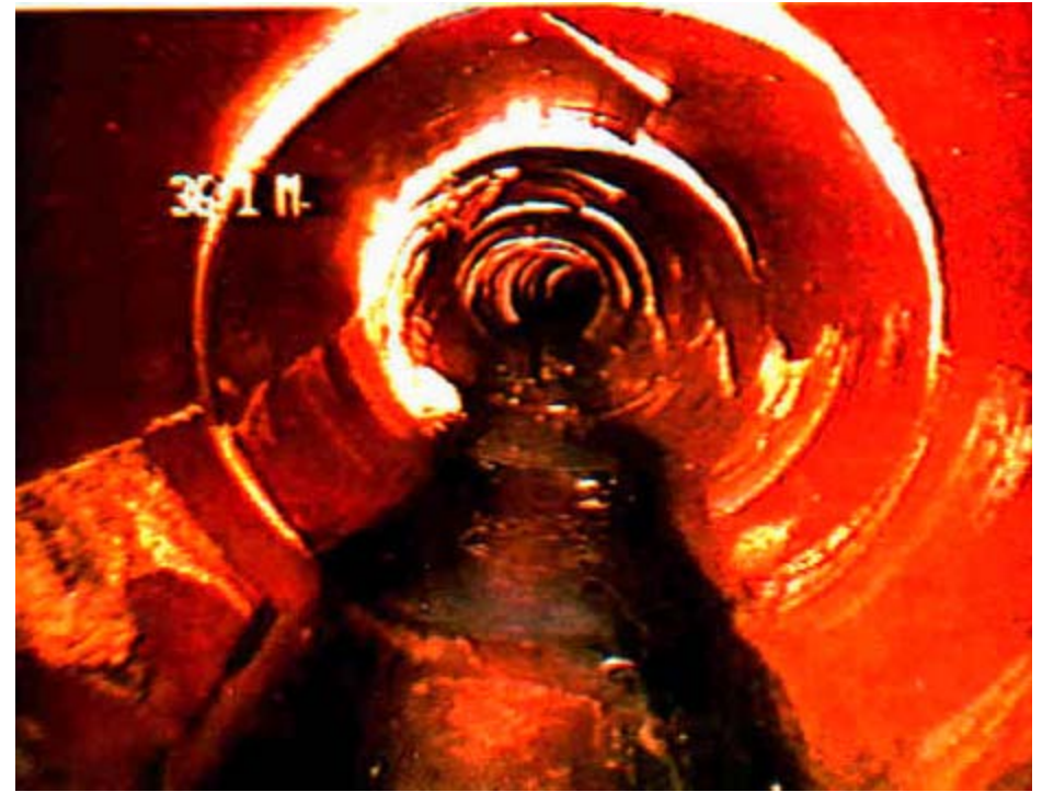
Rigid pipe: Longitudinal fractures: excess moment
