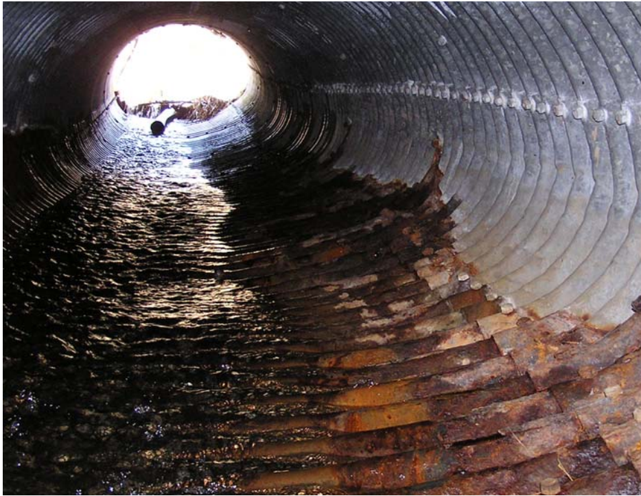
Metal Culvert: Invert and waterline corrosion
