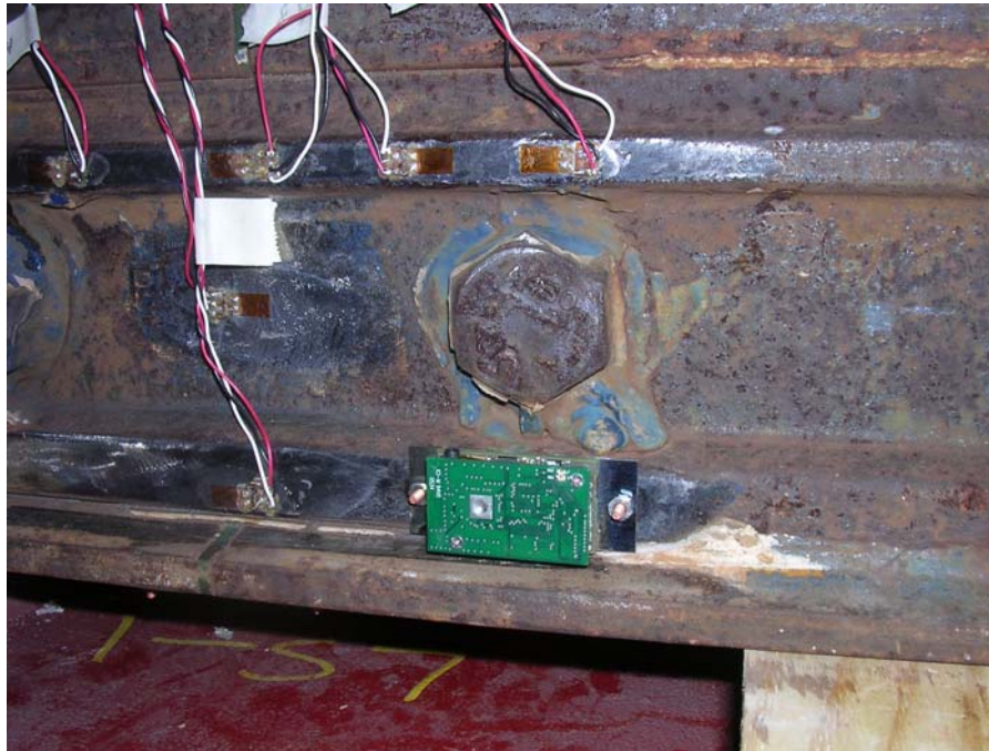
FIGURE 28 Sensor installed on an insulated joint
