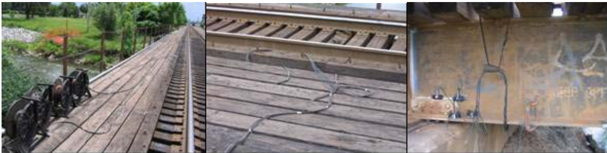
FIGURE 7 An example of cabling required for bridge testing with commercial acoustic emission technology. Left – Four 100-foot BNC cable bundles; middle – multi-channel BNC cable along bridge deck and sub-deck; right – continuation of cable sub-deck with required cable harnessing. It is estimated that wired sensor installation including the wires and technician labor required to install the wired sensors accounts for 30 to 40% of total bridge inspection cost.
