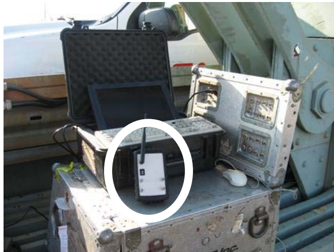
FIGURE 9 Wired and wireless systems shown in CN's Victoria Bridge. The wireless system is shown circled on the metal box that houses the wired system's PC. Shown on top of the metal box are the monitor and keyboard which are required to setup and run the wired system. The wireless MOTE is activated via a remote laptop.
