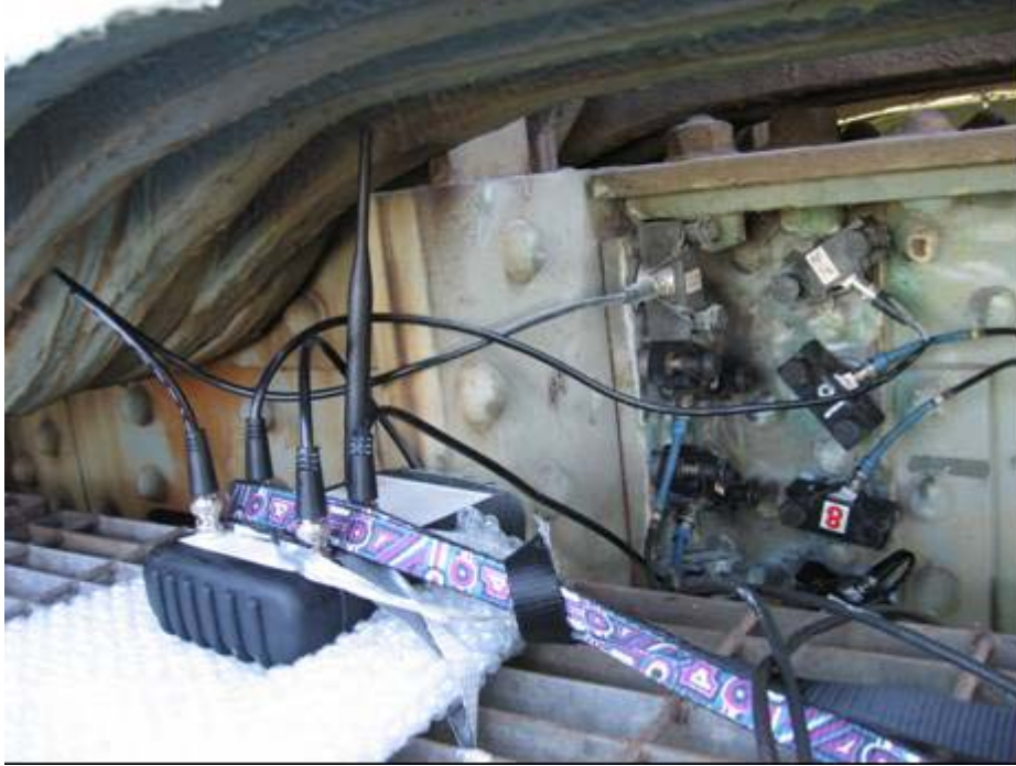
FIGURE 10 Wireless MOTE secured adjacent to the connection angle monitored.
