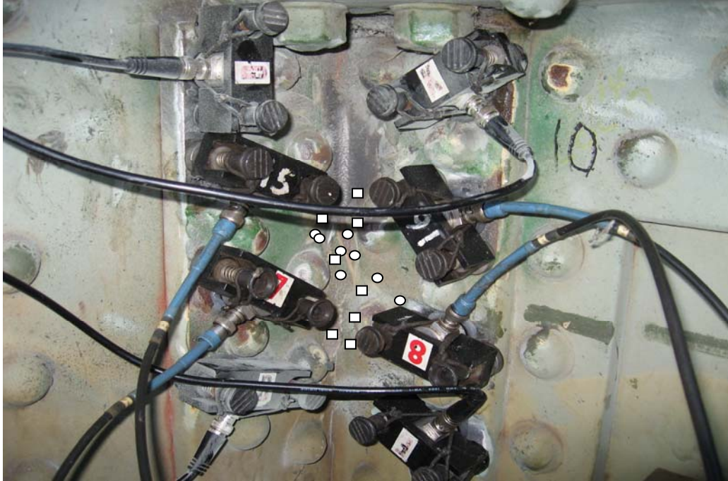
FIGURE 12 Estimated location of wired (circles) and wireless (squares) events showing that all the events are clustered in an approximate 3" x 2" area on the connection angle.
