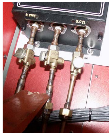
Fig 14 Brake pipe on Shoreliner Cab Car. This interface is fed into the event recorder so SmartSander could be connected here.
