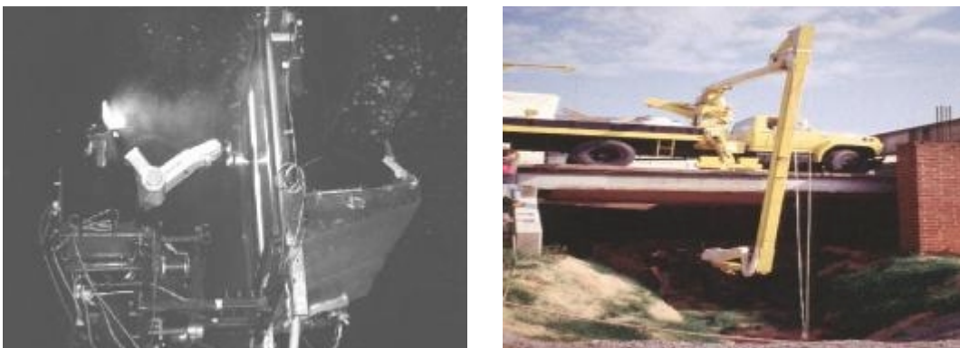
Figure 17 Teleoperated Bridge Paint Removal Machine. (Photo courtesy of Construction Automation and Robotics Laboratory (CARL) at North Carolina State University.)
