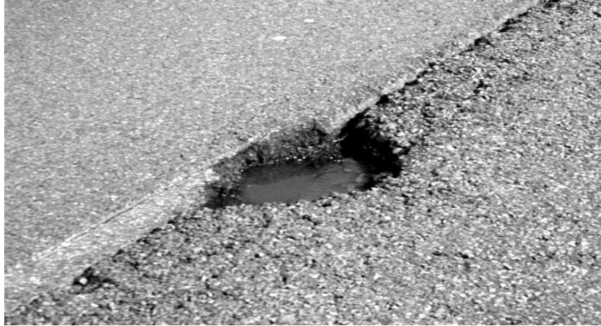
FIGURE 7 Distressed longitudinal joint.
