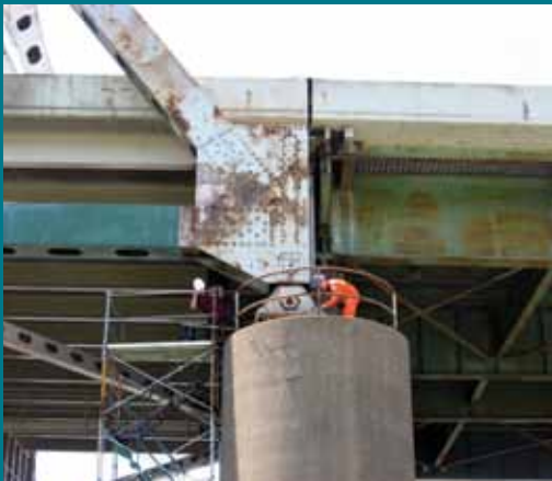
Wireless remote strain monitoring equipment, J.F.K. Bridge, Ohio River at Louisville
