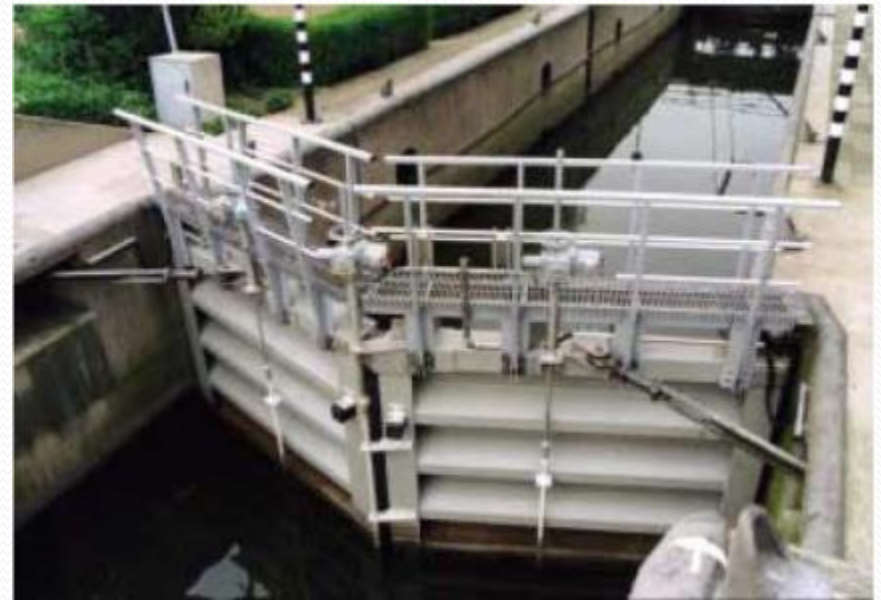
Lock Spieringsluis, Netherlands
