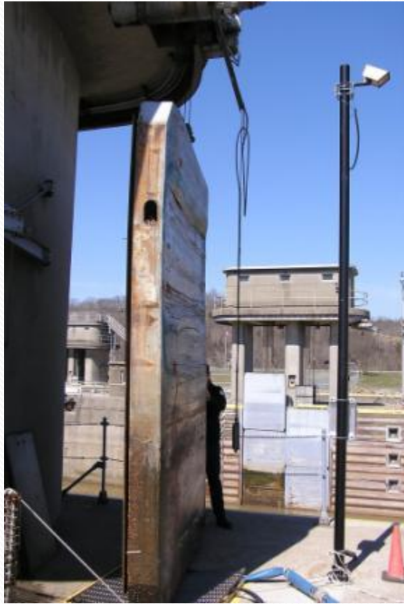
10'x12' steel protection panel with heavy weight & corrosion
