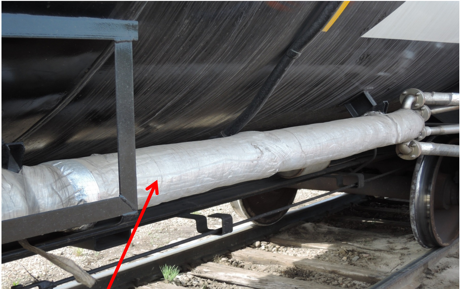
Heat Exchanger/Evaporator LNG to Gas
