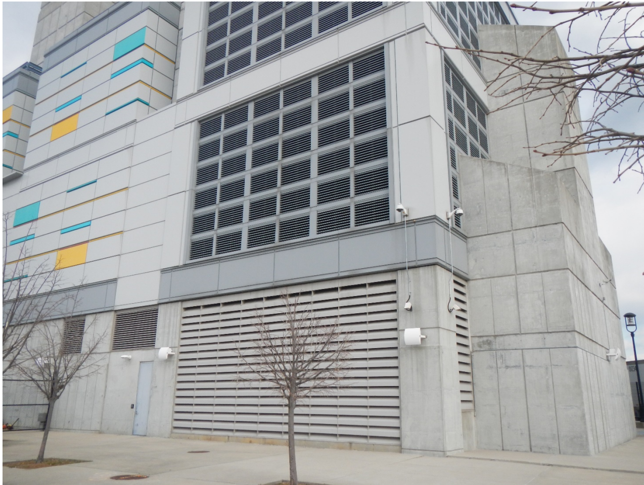
Vent Building 1 – Detail of Air Exchange Vent
