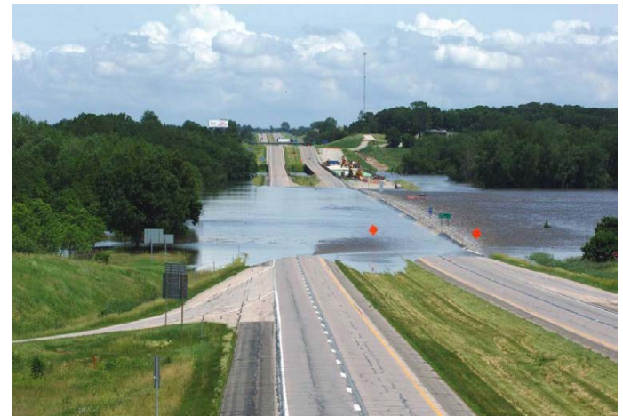
I-80 overtopping at the Cedar River east of Iowa City, June 2008. Photo credit: Iowa DOT.
