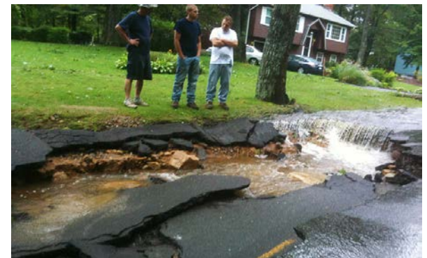
Severe roadway damage during a storm. Photo credit: Foothills Media Group, 2011.
