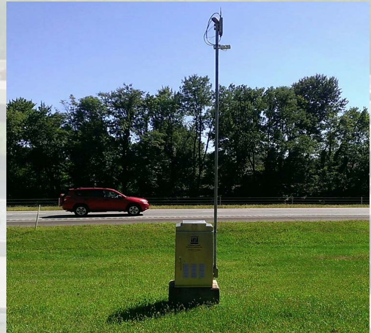
Rest Area WIM Cabinet
