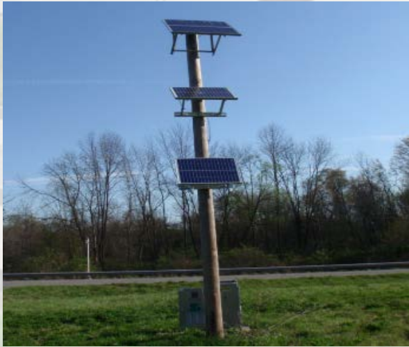
Mainline WIM Solar Panels
